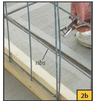
Hog rings tie the panels to each other. Note: Panel ribs should face the outside of the pen.
